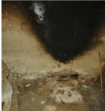
(a) Fire pond
