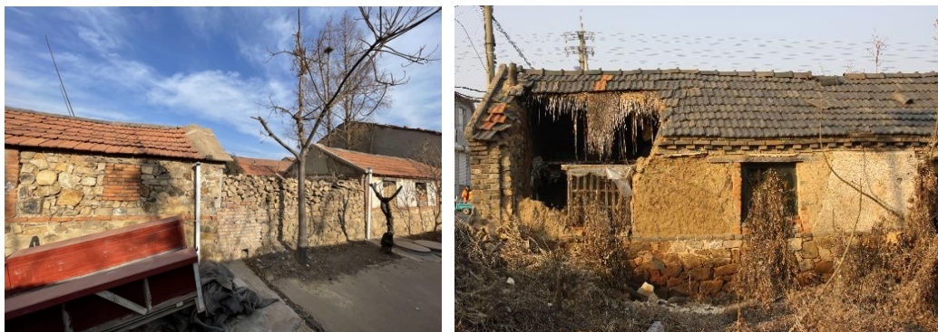
Figure 7.20 The abandoned traditional dwellings
