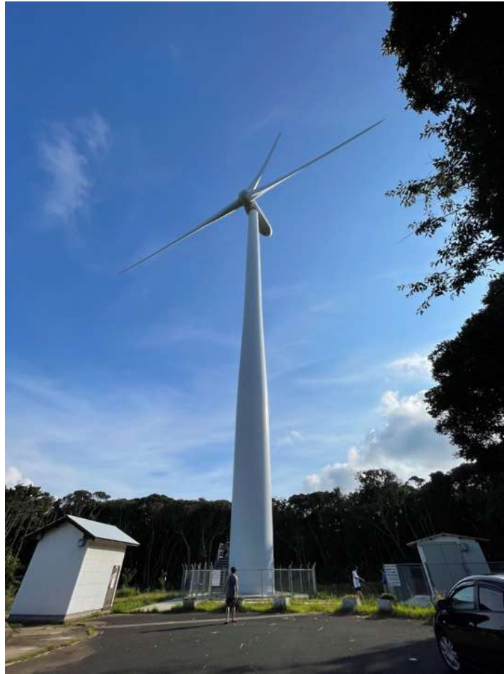
Fig 3. 5 Wind power station in IKISHIMA, Japan (photo by Yafei Wang)
