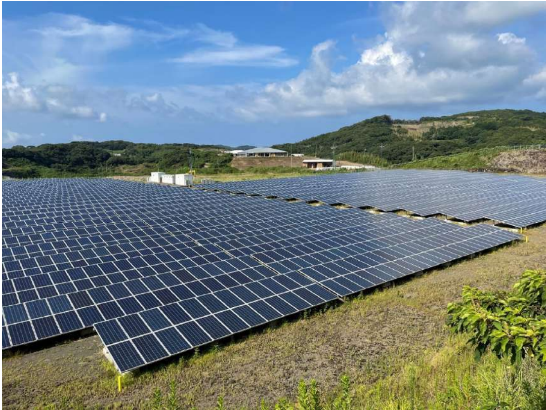
Fig 3. 1 Solar power station in IKISHIMA, Japan (photo by Yafei Wang)
