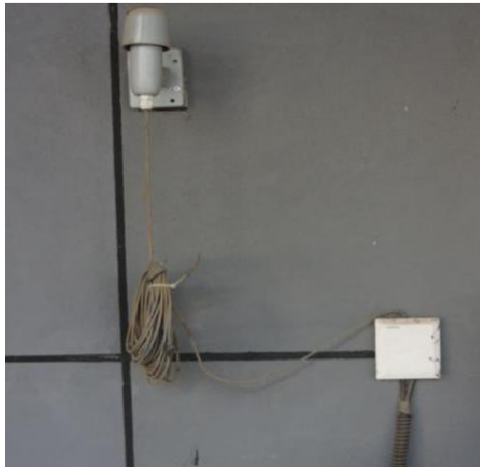
Fig 3-27 Outdoor temperature and humidity sensor
