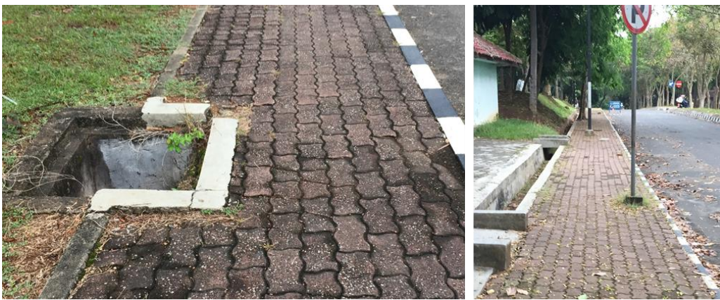
Figure 7.4 Obstruction (hole and pole) on UNILA campus
