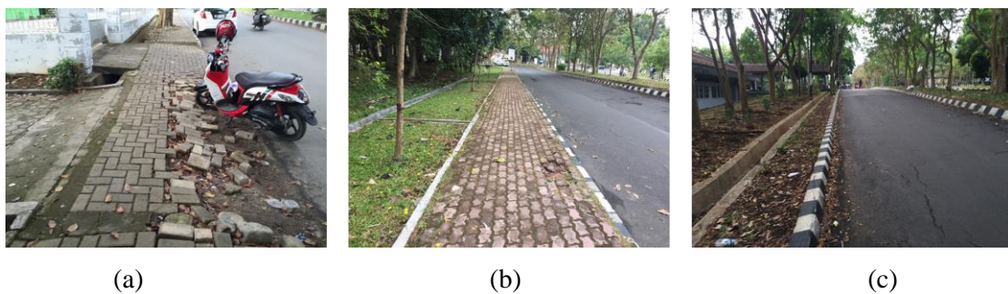
Figure 4.12 Pavement condition: (a) big damage (SW6); (b) small damage (SW7); (c) no pavement (SW5).
