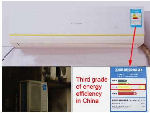
Fig. 8.13 Details of air conditioner used in the experimental building in Sizhai village
