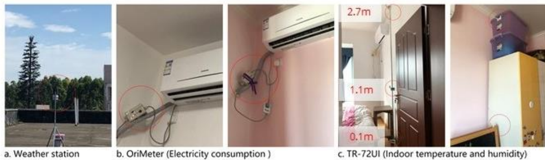
Figure 3-13. Actual layout of the installed measuring instruments.
